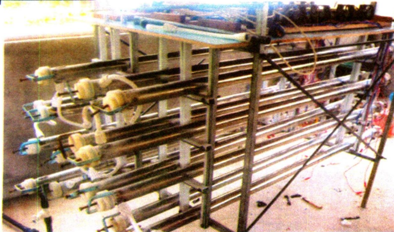
Electro –Coagulation unit at Asokamalagama, Pemaduwa
